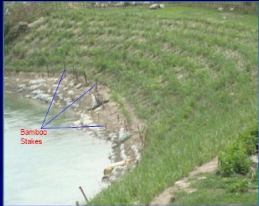
The mattress was pinned to place with the help of bamboo stakes
